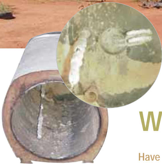
Remains of sacrificial anode. Photographs courtesy of Alison Munroe.
