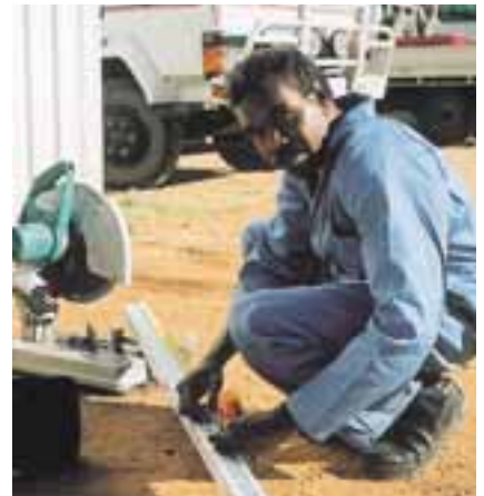
(ABOVE LEFT) NORMAN HAGAN AND MARSHAL DIXON FIT COMPONENTS TO THE JIG. (RIGHT) GIBSON LONG MEASURES STEEL TO BE CUT INTO LENGTHS FOR THE FRAME
